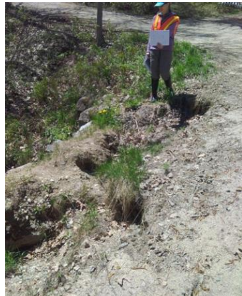
Figure 9. Severe erosion at a culvert
