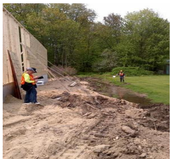
Figure 12. A construction project with inadequate protection of a ditch that leads to the lake
