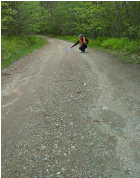
Figure 8. Erosion on the surface of this private road washed into a ditch then into a stream that feeds Lake Pennesseewassee
