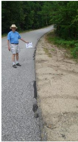
Before: Eroding gravel shoulder at stream crossing culvert.
