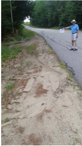
Before: Eroding road shoulders.
