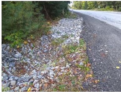
After (above): Rip-rap stabilized ATV trail entrance, “Reclaim” on the shoulder, plunge pool with level lip spreader at the terminus of the ditch before the stream crossing.
