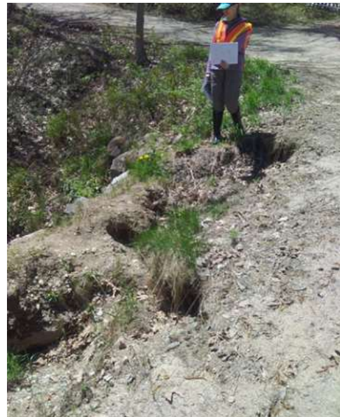
Figure 9. Severe erosion at a culvert
