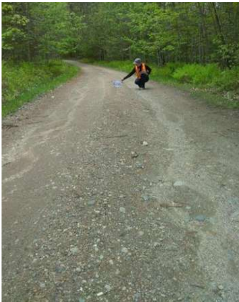
Figure 8. Erosion on the surface of this private road washed into a ditch then into a stream that feeds Lake Pennesseewassee
