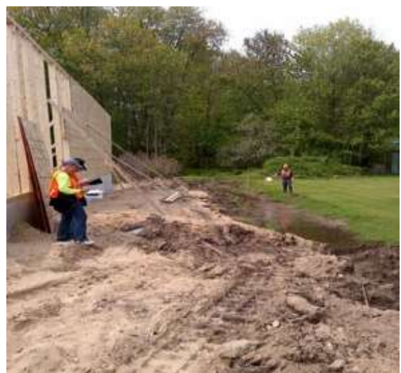
Figure 12. A construction project with inadequate protection of a ditch that leads to the lake
