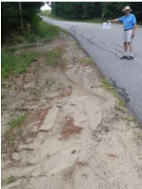
The shoulder along this steep town road erodes into a stream that flows into North Pond.
