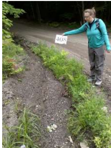
Erosion in the ditch and road surface of this private road washes into a stream and then North Pond.
