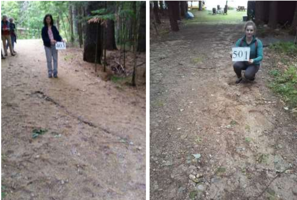
Runoff concentrates on these driveways, and the eroded material washes to the pond.
